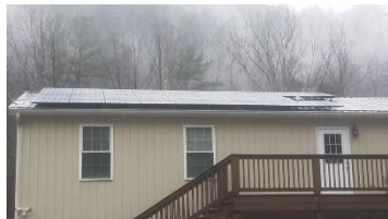
Volunteer House solar panels
